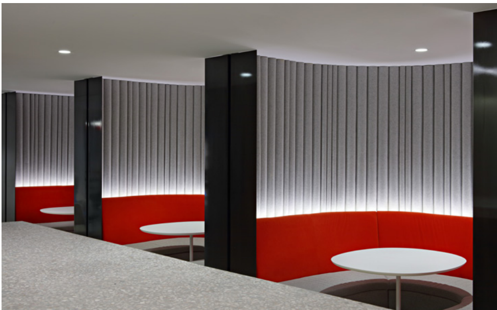
Swell Panels manufactured and installed by DFB | Volunteers of America
